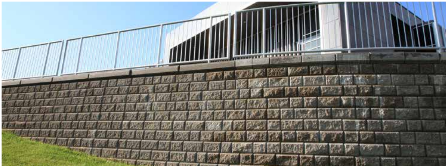
PROJECT: Office Complex Mississauga Rd. Mississauga, ON. DESIGN: RisiStone Engineering. PRODUCT: SonomaStone™ in Natural.
