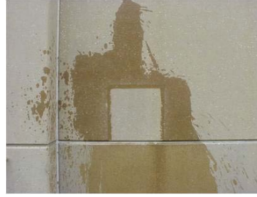
Fig 2. Water sprayed on wall shows the 2'X2' area does not absorb any water
